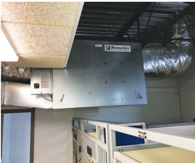
Installation of RenewAire ERV at Broome County (N.Y.) Humane Society
