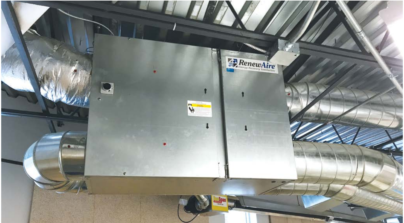
Installation of RenewAire ERV at Broome County (N.Y.) Humane Society
