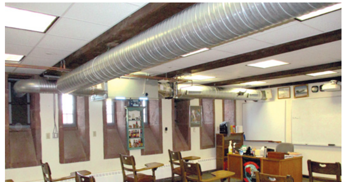
The ceiling was the installation location for the ERVs and ductwork to keep them out of the way.
