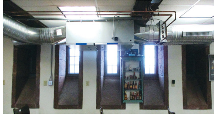
The team placed intake/exhaust vents in windows to maintain the building infrastructure. RenewAire ERVs are simple and flexible to install, and can adapt to space restraints.
