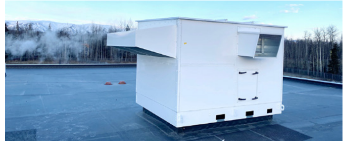
The sustainable mechanical HVAC design features dedicated outdoor air systems (DOAS) with energy recovery and packaged rooftop units (RTU) with heat recovery.
