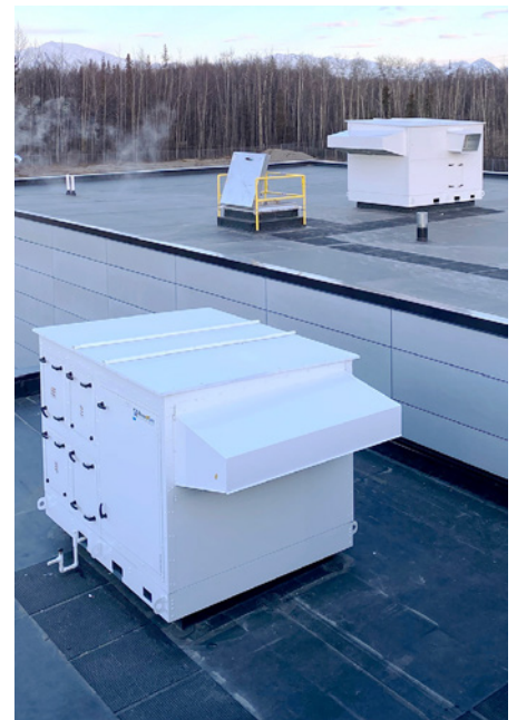
The two DN Series DOAS units provide 3,000 CFM and 1,700 CFM of 100% outdoor air in the facility's 3,100 sq. ft. garage and the 750 sq. ft. evidence room.
