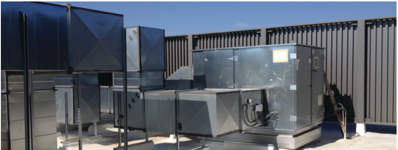
Rooftop installation of RenewAire ERVs at GCU Image courtesy of MSA Engineering Consultants
